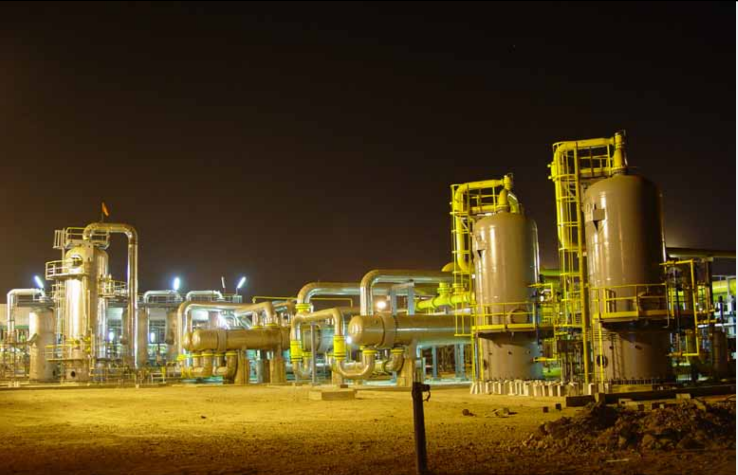
Qadirpur gas processing plant
