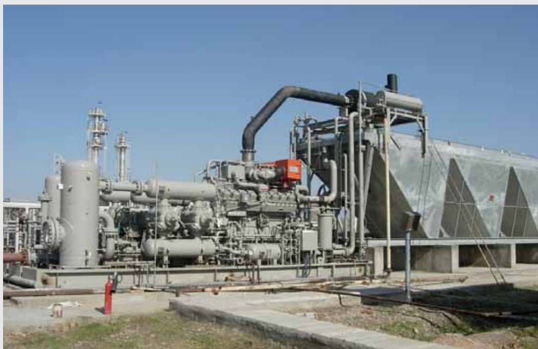
Gas compression recently installed at Chanda field
